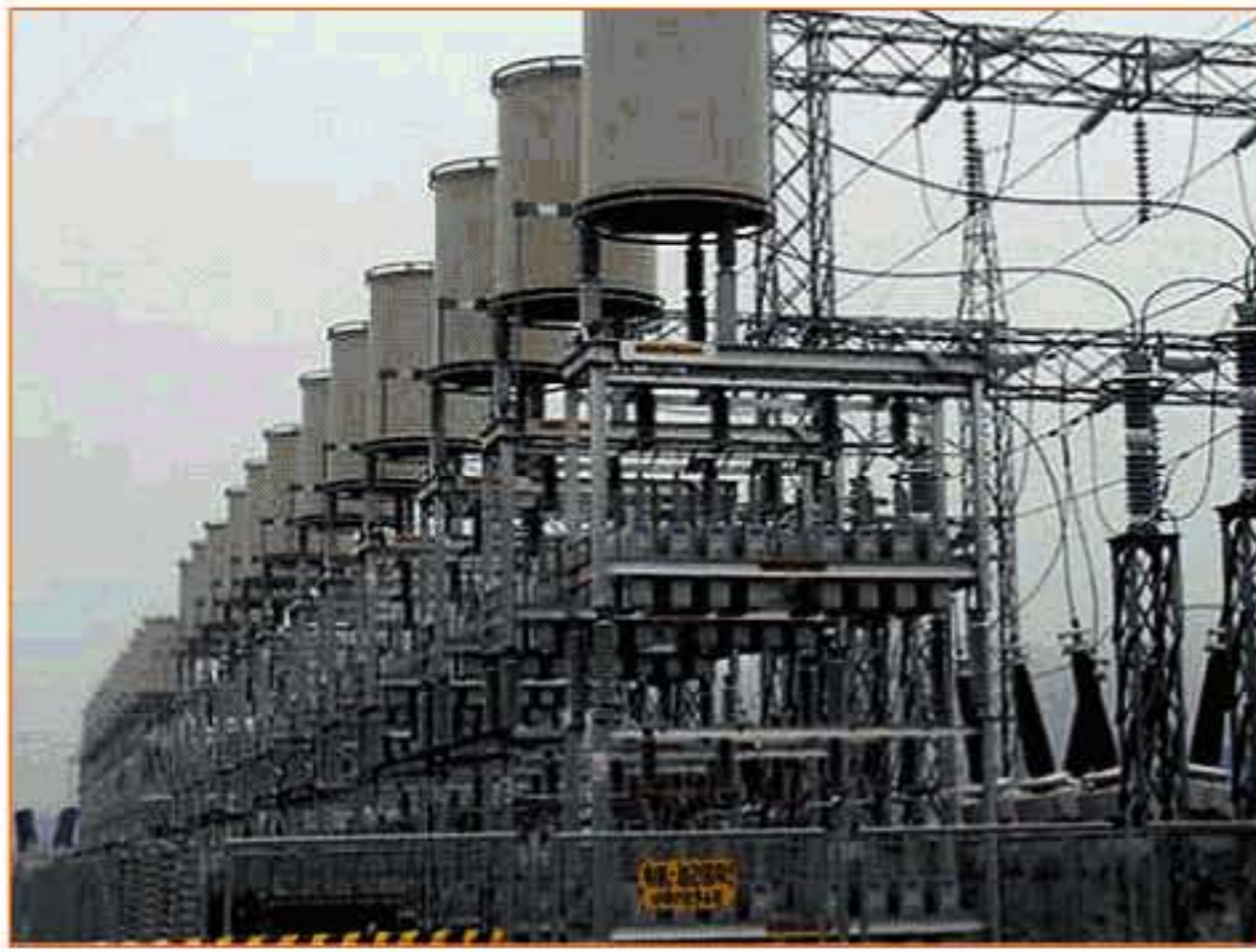
Eight, 50 Mvar, 154 kV Banks in parallel
